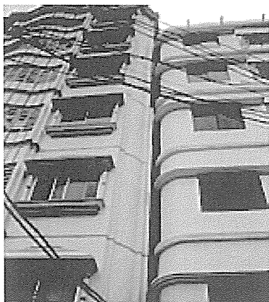
Tilting of 6-story building in Rajshahi (5-Jul-2008 quake)
