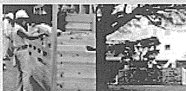
Left: Laying out the wooden-blocks Right: The wooden building with IIS building in the backdrop
