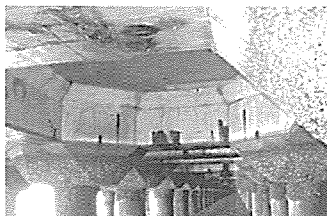
Deterioration of pier due to salt attack
