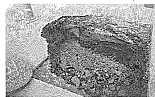
Cave-in in road due to the deterioration of underground pipe
