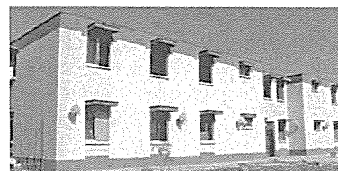
Top: School at Los Molinos, Ica. Note that columns in the 1st and 2nd floor are either not aligned or interrupted. Bottom: Hospital at Pisco, where 80% of the houses were affected, suffered no damage.
