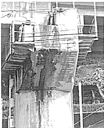
Corrosion of steel due to the use of sea sand as fine aggregate
