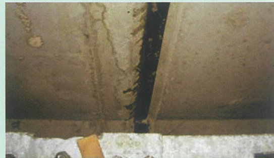
Observed deterioration inside box culvert structure
