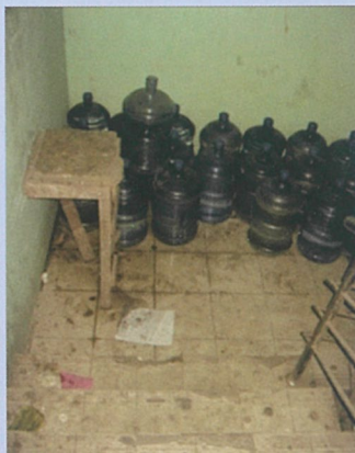
Blocked emergency exit of commercial building
