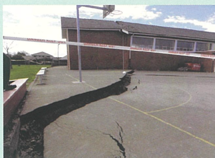
33 cm vertical offset observed at St. Paul's Church, Dallington (Cubrinovski et al.)
