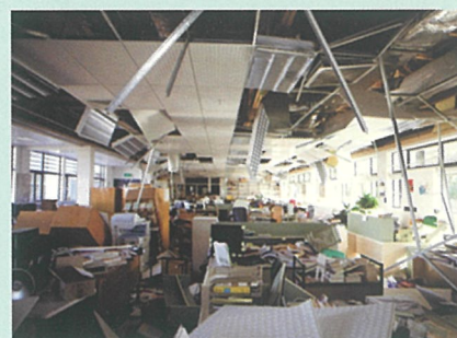
Damage to ceilings and contents (photo: Giacomo Paganotti)
