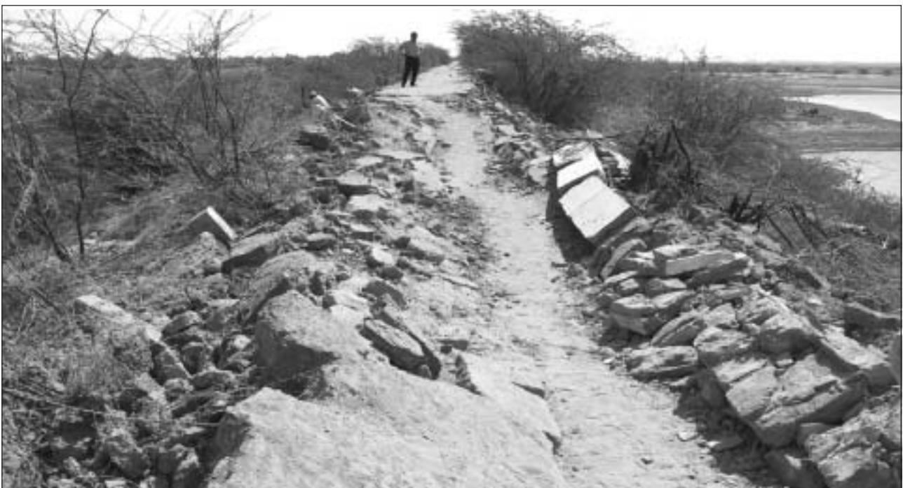
Cracks along the crest and vertical settlement of the Suvi dam damaged during the January 26, 2001 Bhuj earthquake (Mw 7.7) in Gujarat, India (courtesy: JSCE, Japan)
