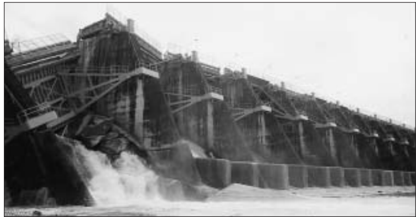
Shi-Kang water supply weir damaged during the Chi-Chi earthquake (Mw 7.5) of September 21, 1999 in Taiwan (courtesy: K. Meguro)
