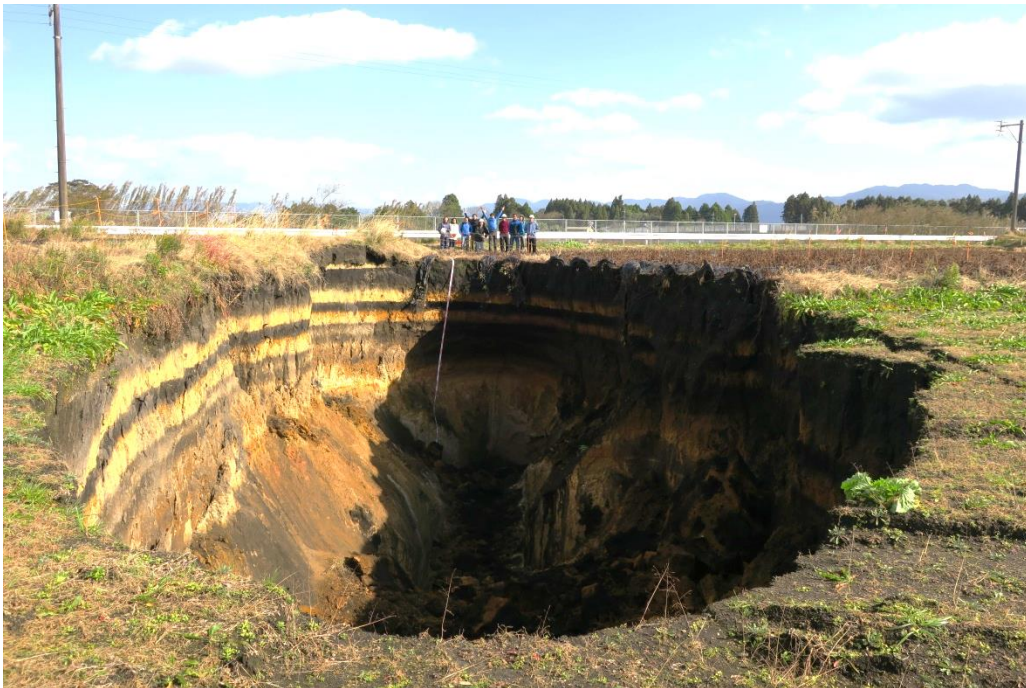
Sinkhole in Miyakonojo
